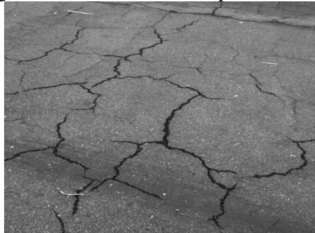
Figure 3: Formation of cracks on bituminous road surface.
